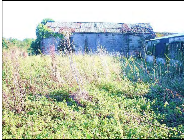
Photo 153: Rear northwest elevation of ‘B4’ and ruderal vegetation in the northwest area of ‘Parcel 13’.
