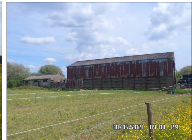
Photo 35: Rear northern elevations of ‘B12’ and ‘B13’ and poor SI grassland with view from the north towards the south.
