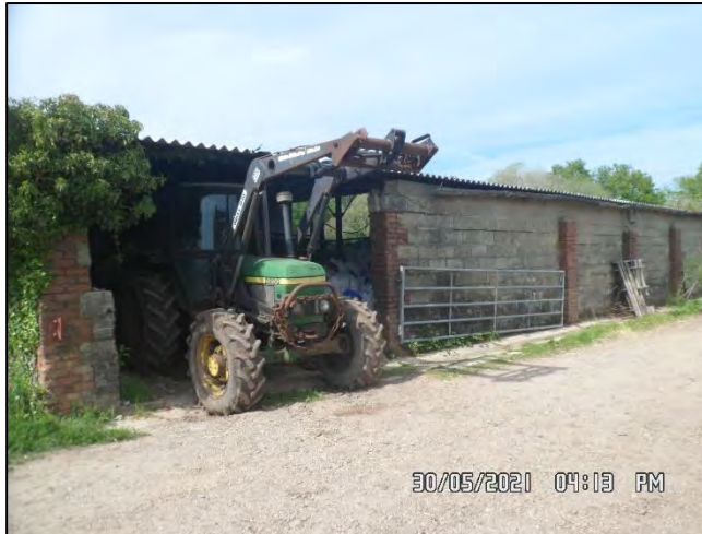
Photo 37: Southern elevation of 'B12' with view from the southwest towards the northeast.
