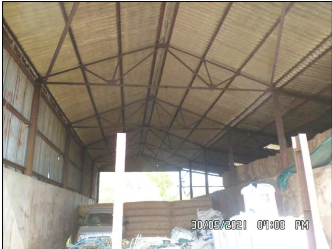
Photo 36: Internal of 'B12' in the southeast of 'Parcel 3' with view from the south towards the north.
